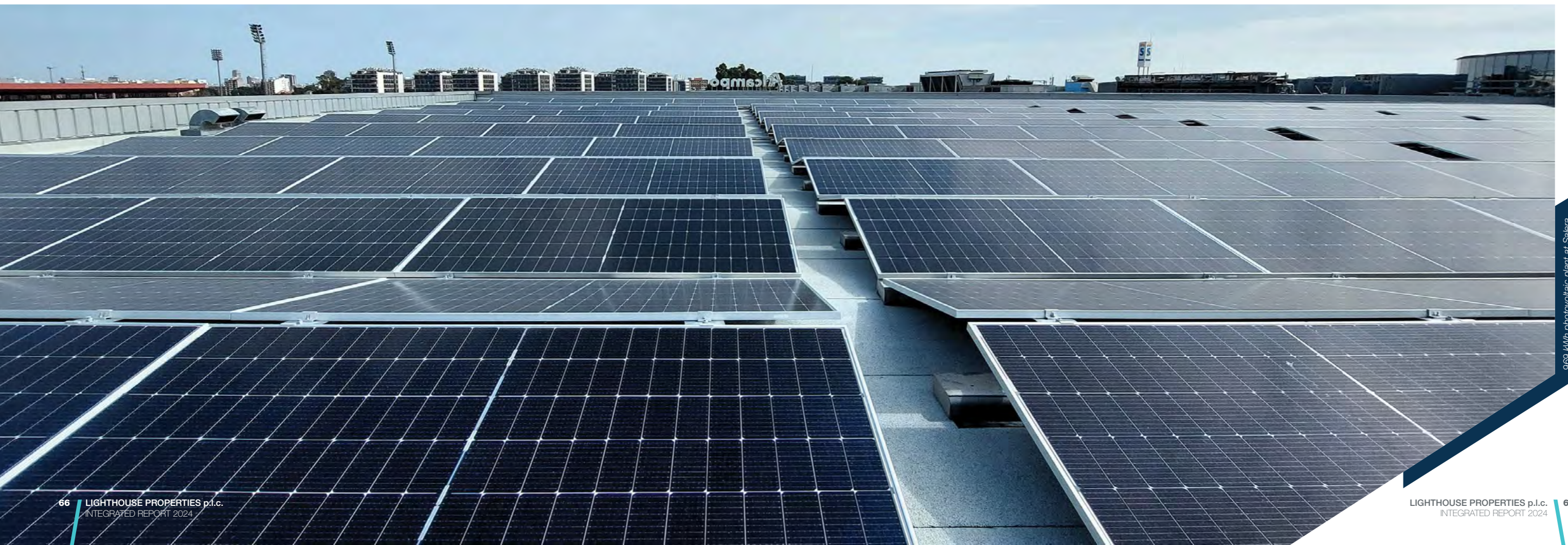
969 kWh photovoltaic plant at Salera
