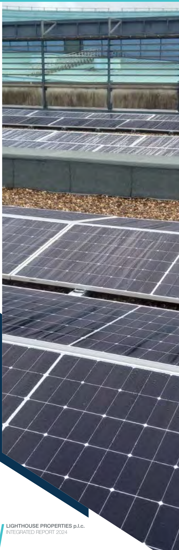
PV Installation at Forum Coimbra
